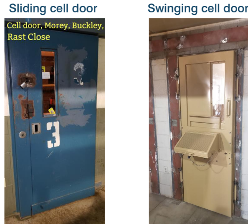
Figure 4 Department’s old sliding door and new swinging door
