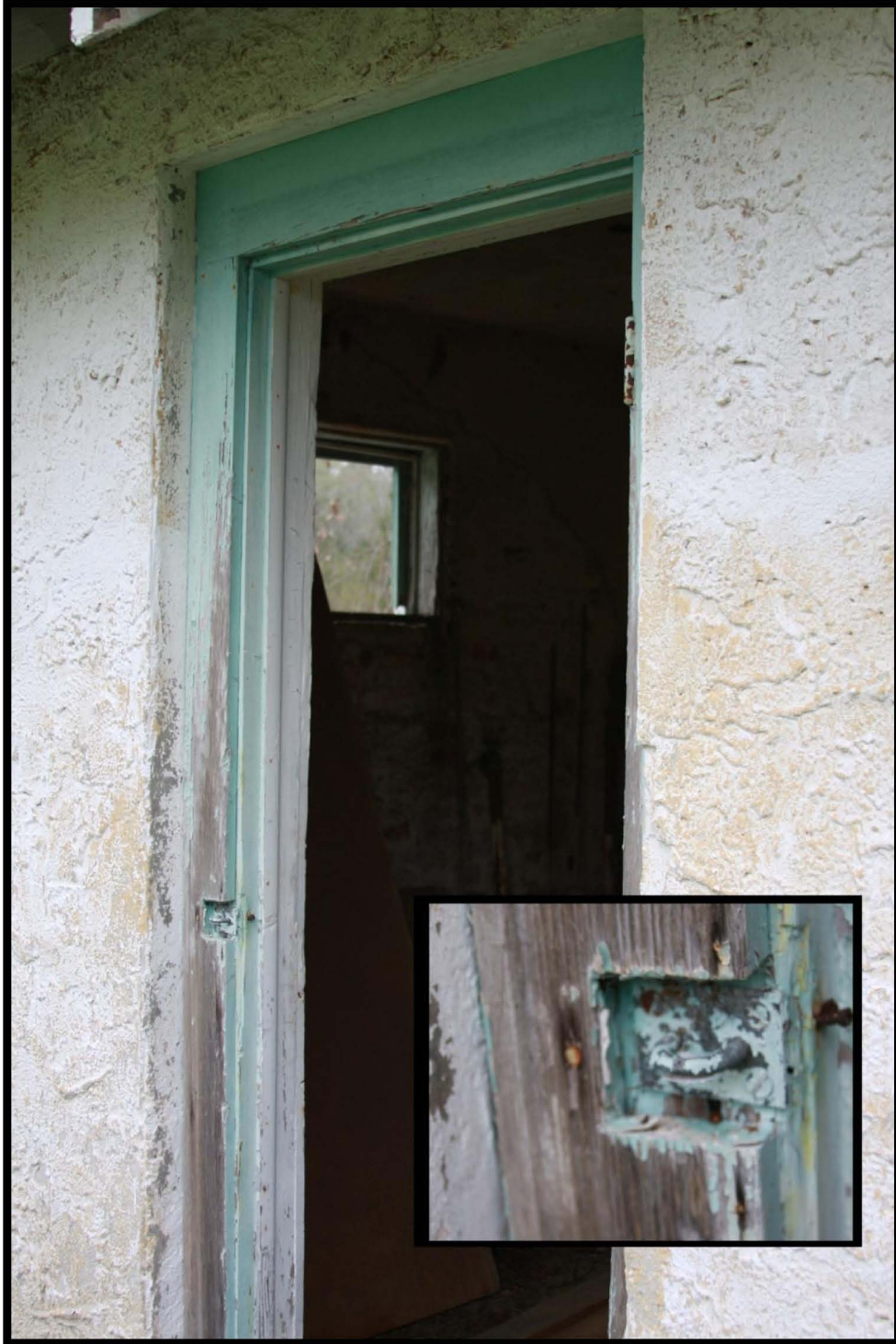
Figure 11. Door frame of confinement cottage showing modification to door when building was converted from storage to confinement cottage and later to the farm manager's office. The door was modified to swing outside, rather than inside. The small window in figure shows former outside latch for lock.
