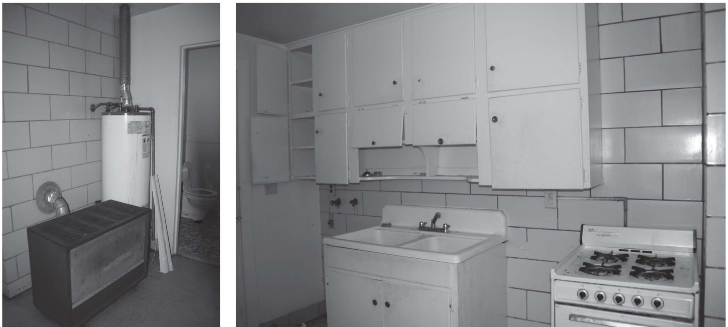
Figure 9: Unit That the Athens Housing Authority Plans to Renovate with Recovery Act Funds
